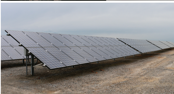
(Above) Brig. Gen. Timothy P. Williams, the Adjutant General of Virginia, prepares to symbolically turn the switch to send power from the newly-constructed solar array to the administrative and classroom facilities at the 183rd Regiment, Regional Training Institute at Fort Pickett (Photo by Capt. Andrew J. Czaplicki, Virginia Guard Public Affairs) & Solar Array at Fort Pickett
